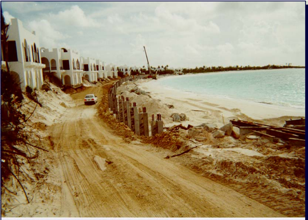
HURRICANE RAVAGED SHORELINE RESULTED IN UNDERMINED BUILDING FOUNDATIONS AND REQUIRED THE INSTALLATION OF OVER 1000 LINEAR FEET OF PRE-CAST CONCRETE SEAWALL AND THE REPLACEMENT OF LOST FILL MATERIAL.
